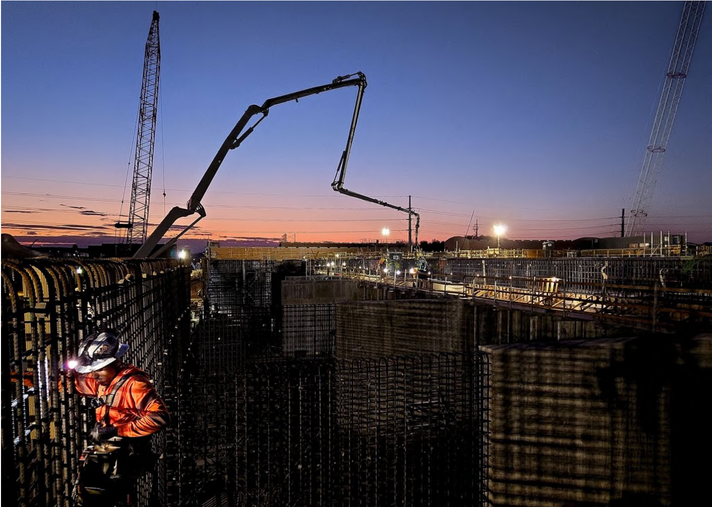
The Southern Nevada sunrise as expansion work continues at the Flamingo Water Resource Center
